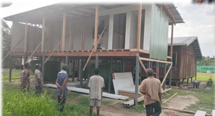
The construction at the end of 6 weeks, after four weeks of independent work by the local team
