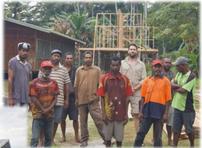
The construction at the end of the two weeks of the two-man Rotary Australia World Community Service Team project
